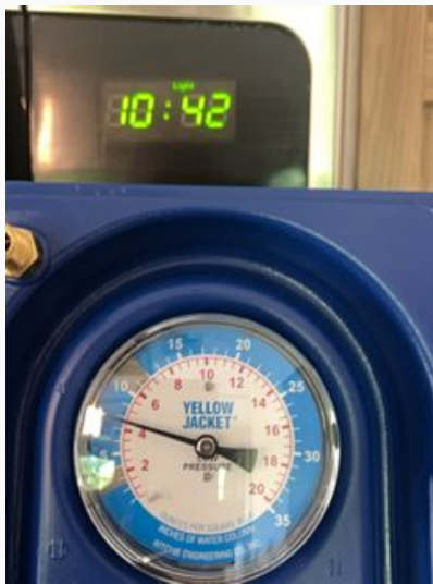
Start time: 10.42 - 8" Water Pressure
