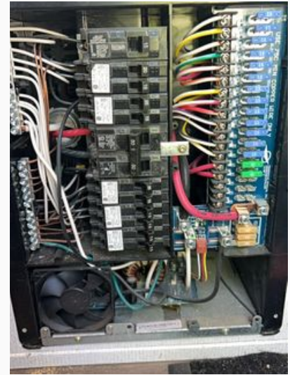
Inside electrical panel
