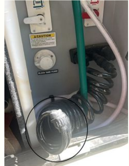
No shower head installed
