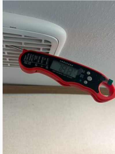
Air Inlet temperature 79.8F
