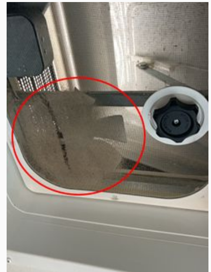
Main bathroom ceiling fan
