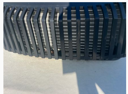
Air Conditioner Coils
